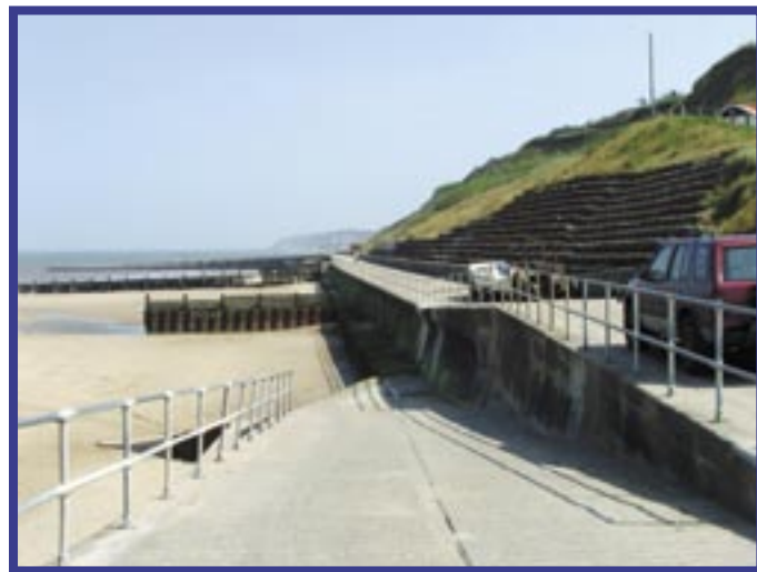
Coast protection at Overstrand, North Norfolk
